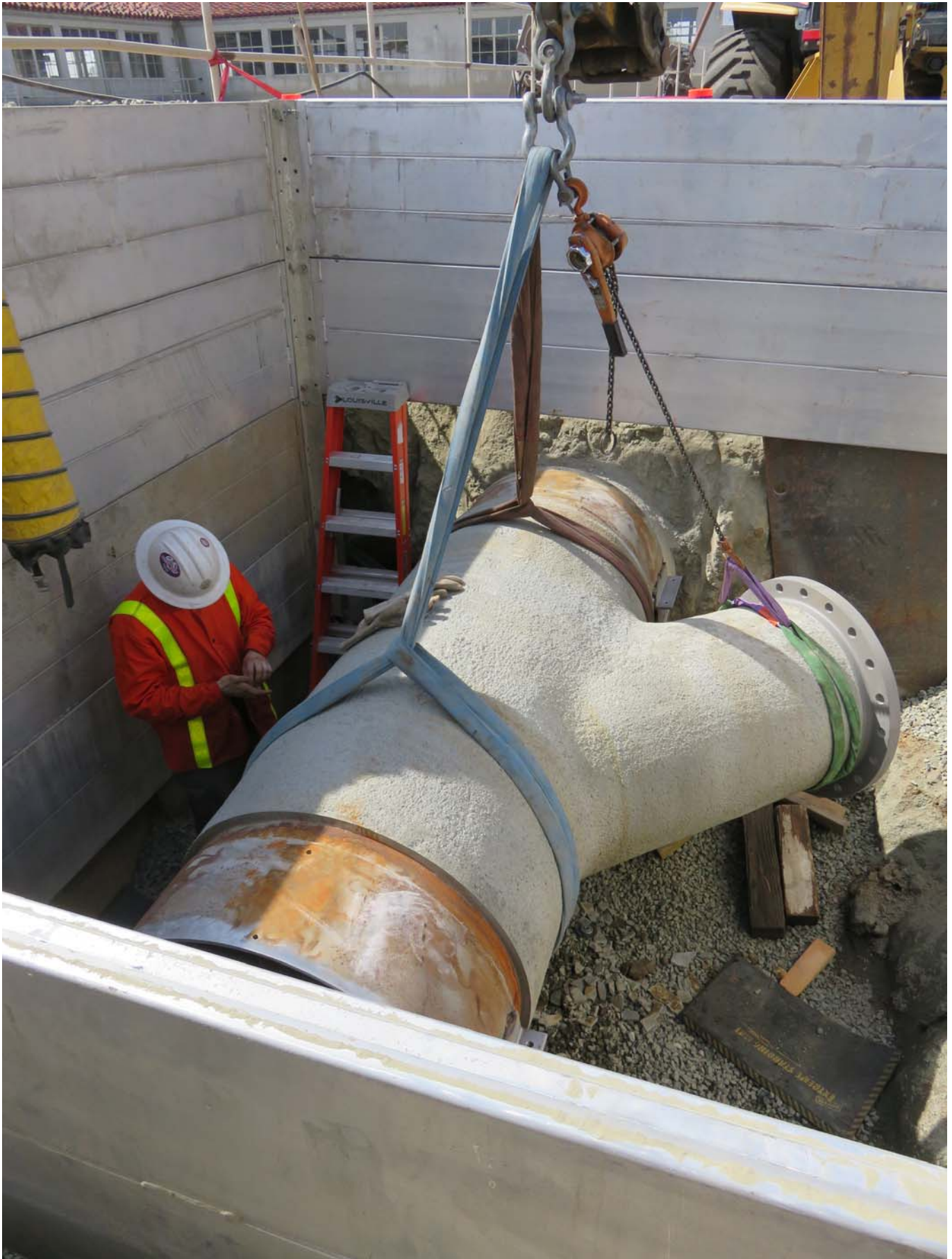
Pipe-tee installation at Weymouth Plant as part of the Ozone Retrofit Project.
