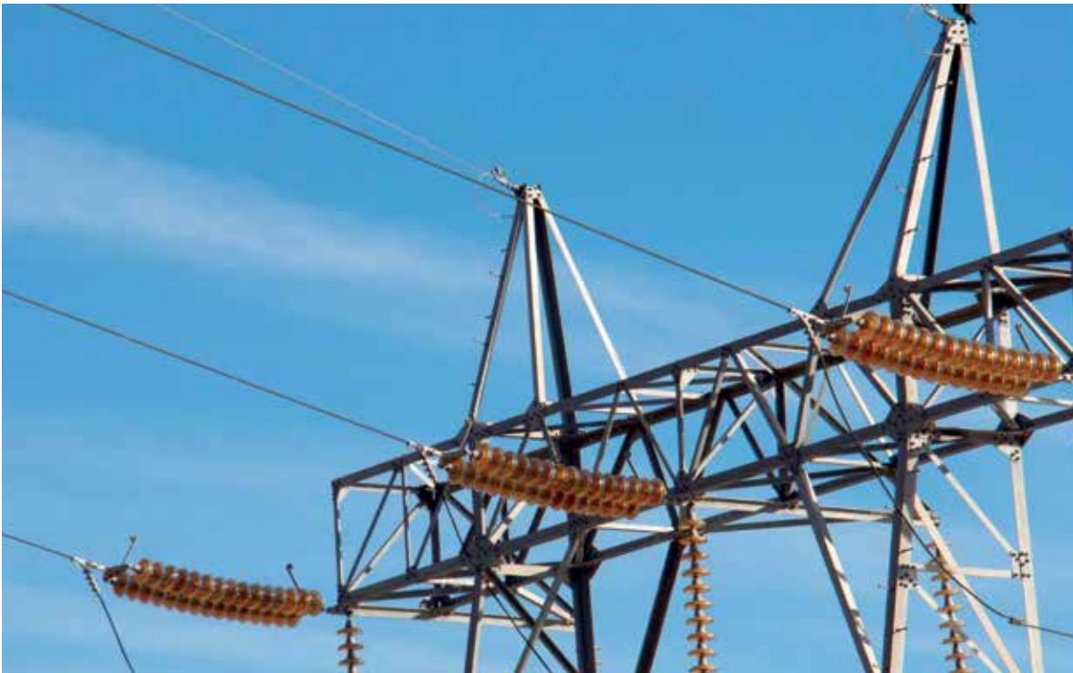
Electrical transmission lines along the CRA
