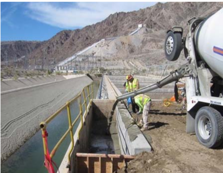
CRA sand trap rehabilitation work at Hinds Pumping Plant during 2016 CRA shutdown.
