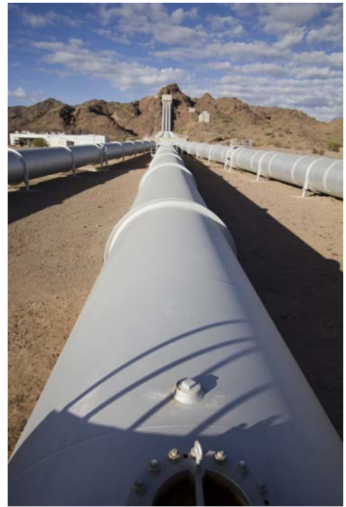
Penstocks at Gene Pumping Plant delivering Colorado River Water Supplies
