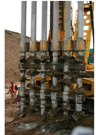
San Pablo Dam Seismic Upgrade prevents dam failure in the event of an earthquake.
