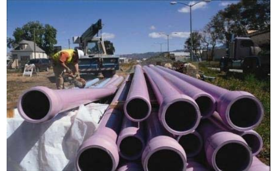
East Bayshore Recycled Water Project supplies water for landscape, industrial, and commercial use.
