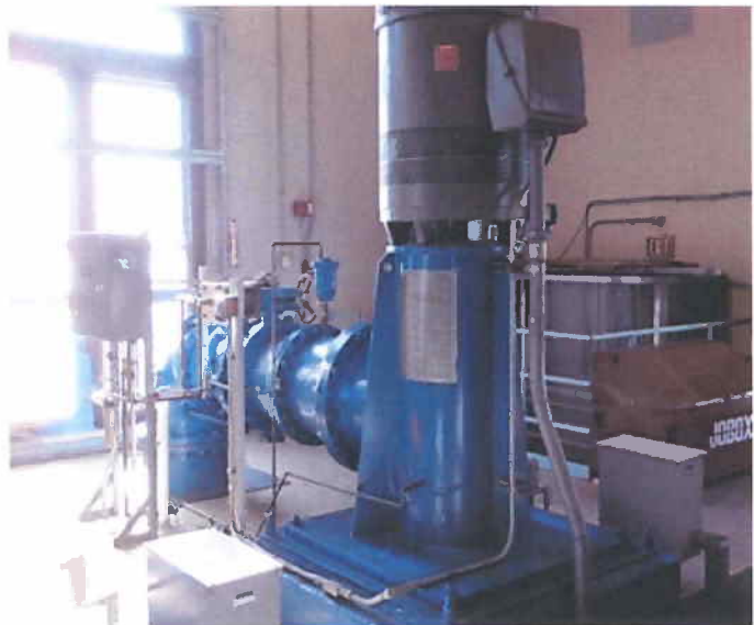
Pump 1 (constant-speed) motor to be replaced with new pump and VFD.
