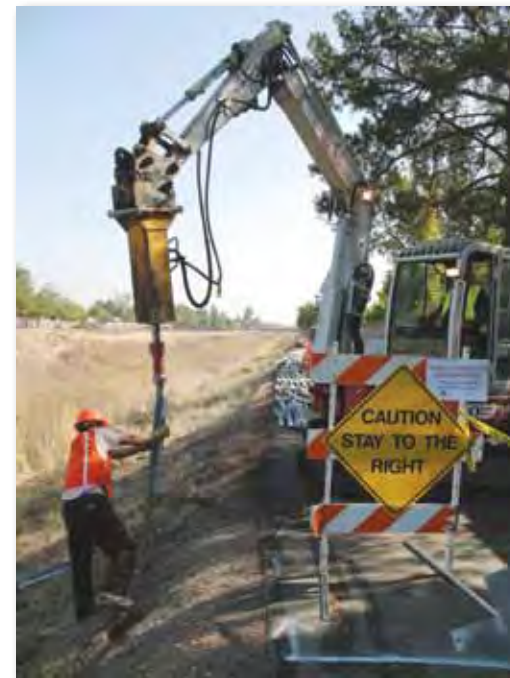
A pilot project launched along Arroyo Mocho in 2009 is evaluating the effectiveness of a new slope stabilization technology. Hundreds of steel plates were welded to 6 1/2-foot-long steel piles along 1,000 feet of tightly constrained channel slope.
