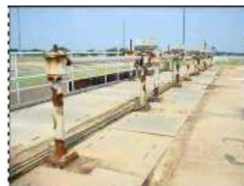
Photo 6 - Pre-aeration Tank Slide Gates
