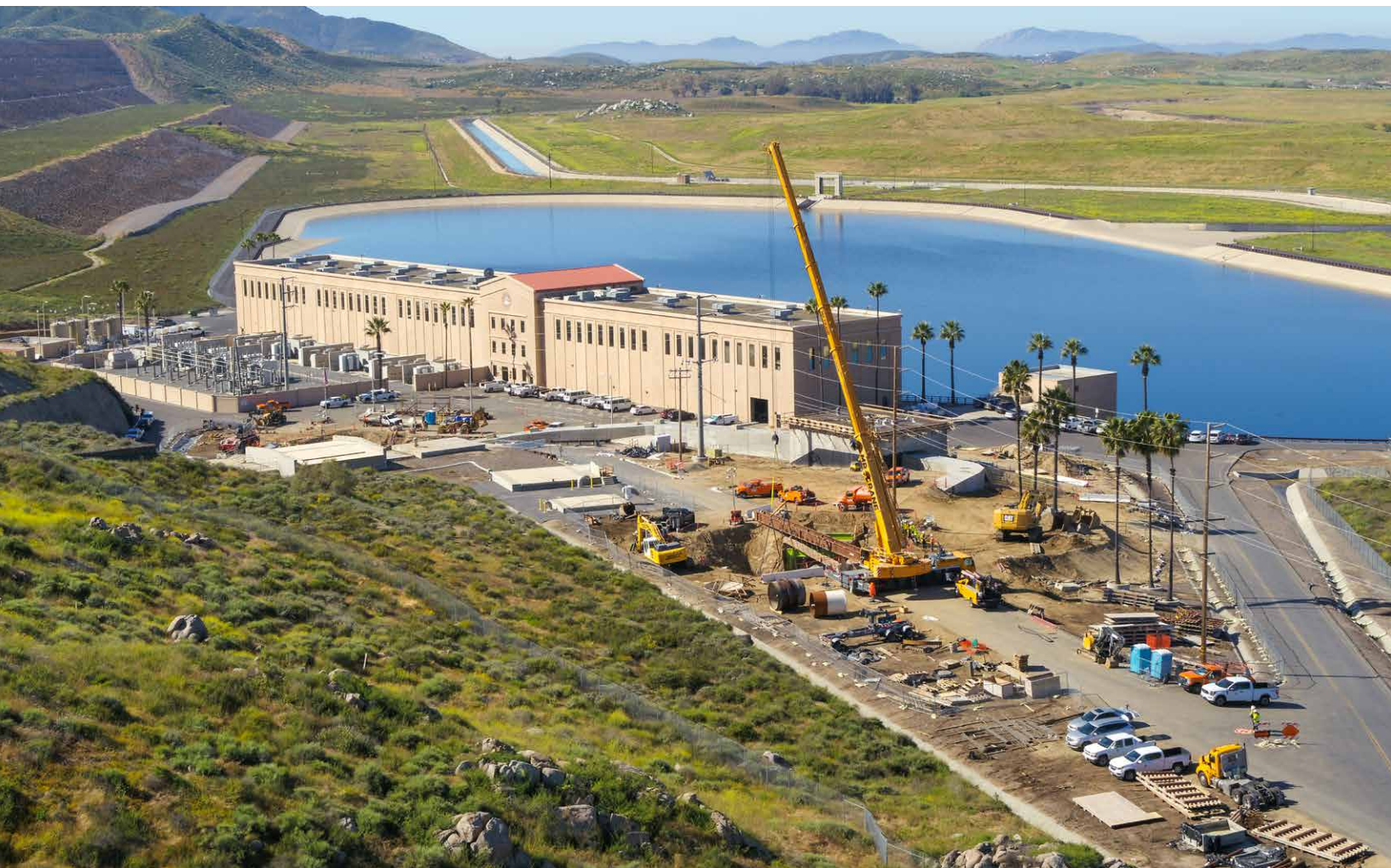
The Wadsworth Pumping Plant Eastside Pipeline Intertie project brings greater flexibility to Metropolitan's delivery system.
