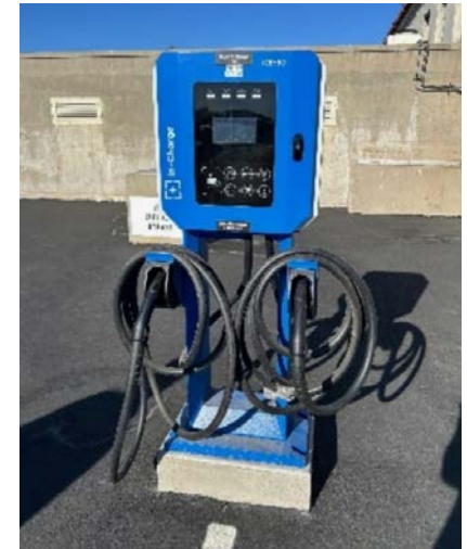
Weymouth WTP Pilot Charger
