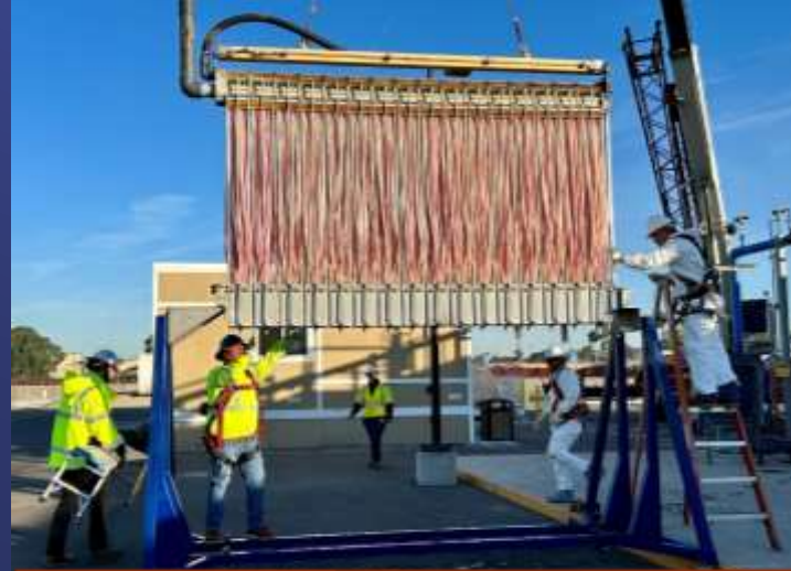
MBR Membrane Maintenance
