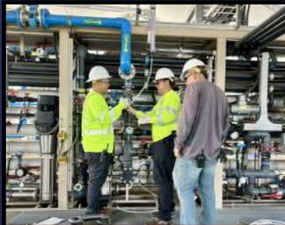
New Chemical Tubing
